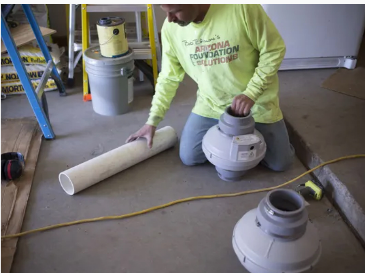
Terry Henry puts together a ven fan, April 15, 2015, on an Arizona Foundation Solutions job in Peoria. (Photo: Mark Henle/The Republic)
