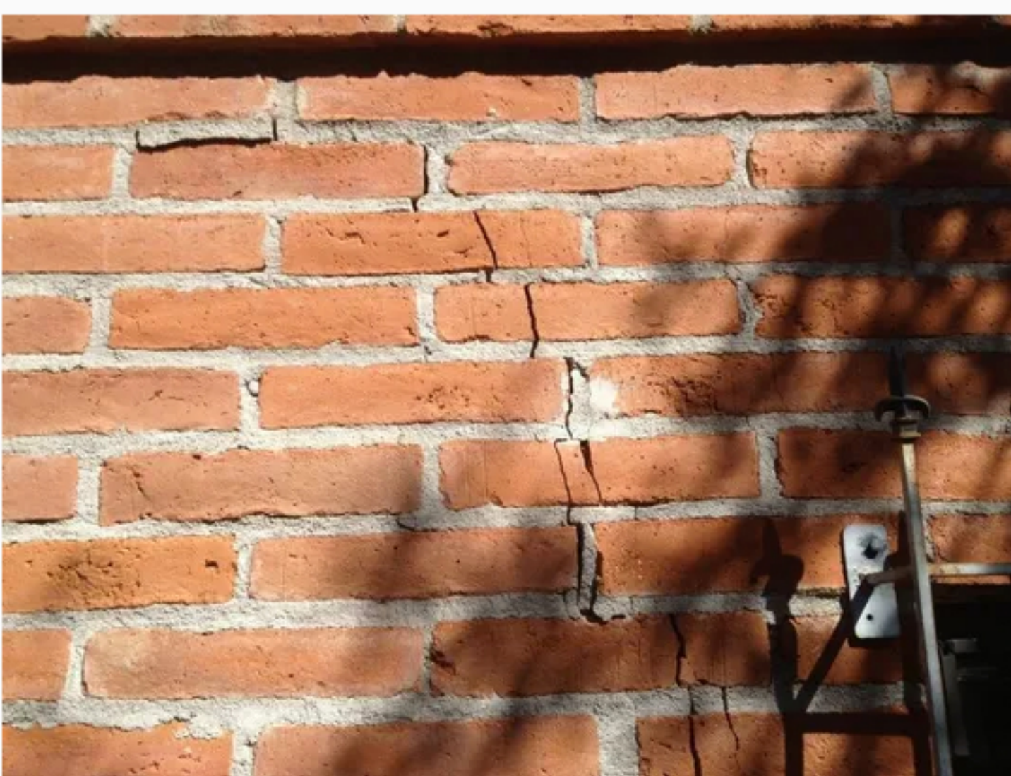
After work was done to secure the foundations of the house, the crack is much smaller. Now the seams between the bricks can be refilled. Credit: Arizona Foundation Solutions. (Photo: Handout / Arizona Foundation Solutions)
