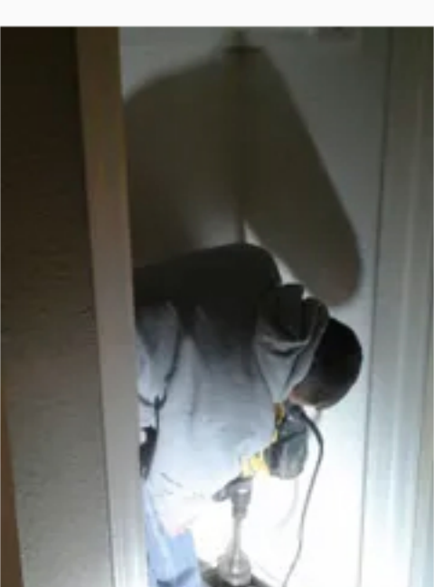
The pipe can be run from the roof down through a closet where it will be out of sight in the home. (Photo: Handout / Arizona Foundation Solutions)
